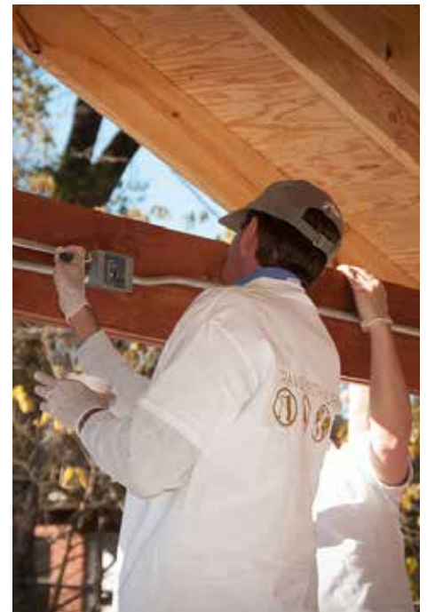
Hilton Worldwide Team Members work on construction projects during Global Week of Service, November 2012.
